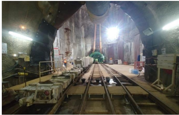
Fig. 11: View from base of drop shaft with the setup of rolling stocks tracks and logistics shaft and tunnel
